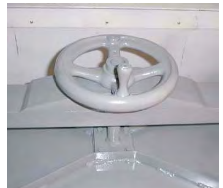
INCORRECT! Handle in front position.
