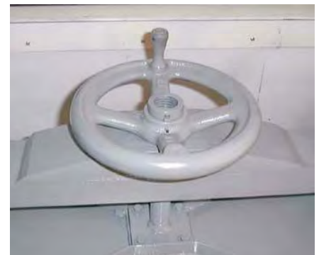
INCORRECT! Handle in back position.
